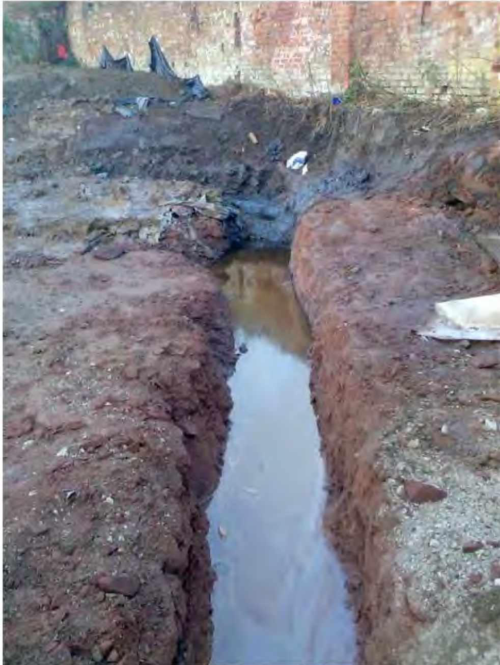
Photograph 5: Hydrocarbon impacted soils and water within foundation excavation.
