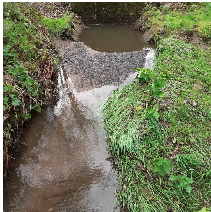
Figure 2 – Partially Blocked Outlet Drain
