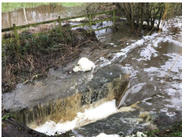
Figure 3 - Mill Brook at the High Street Bridge. 28/01/21 (note that this was taken a week after the event when water levels had subsided)
