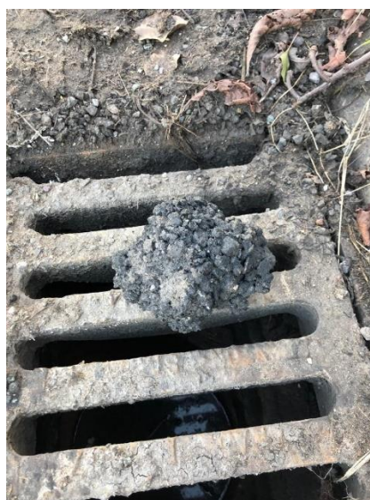
Figure 2 - Road Gulley following Clearance after Storm Christoph
