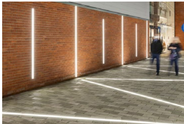
Rochdale Riverside incorporates lighting within the surfaces of the floors and walls to highlight key routes at night-time
