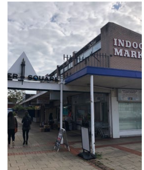
Poor condition of the indoor market
