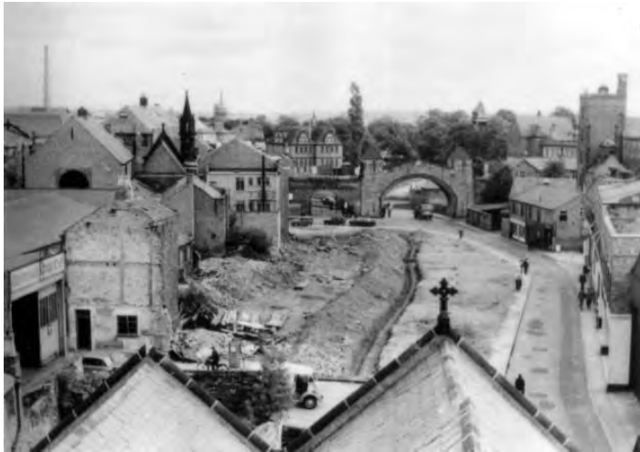
Pepper Street being widened for the ring road: The Newgate far centre.
