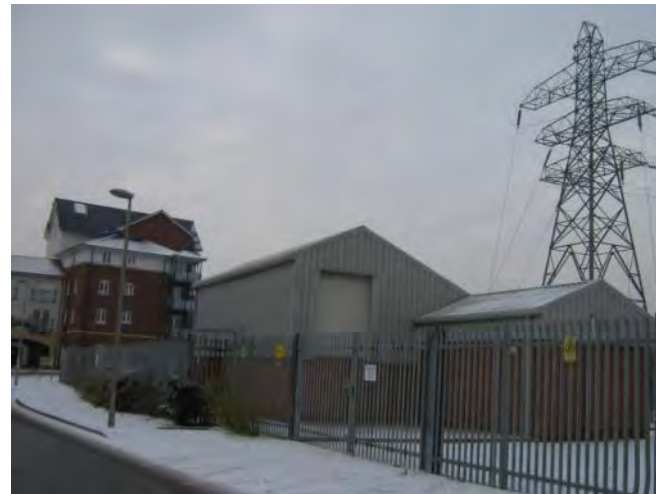
Substation on Sadlery Way
