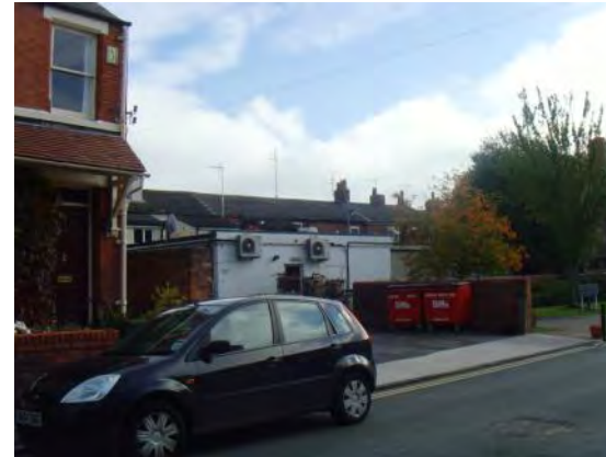
Chiller unit on Derby Place
