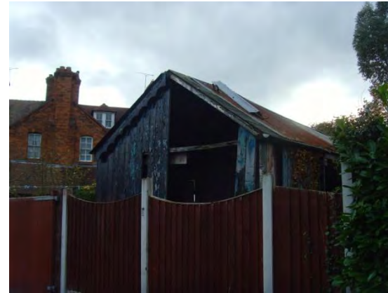
Dilapidated shed at Dyreham
